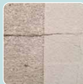
Cement Plaster Higher Drying Shrinkage 0.1%
